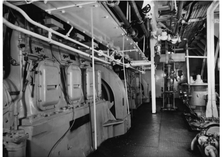
Looking aft on outboard side of generators. Workshop and generator pumps on the right.
