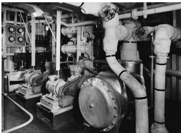
Refrigerator compressors and auxiliary condenser, situated in starboard corner at engine room flat level.
