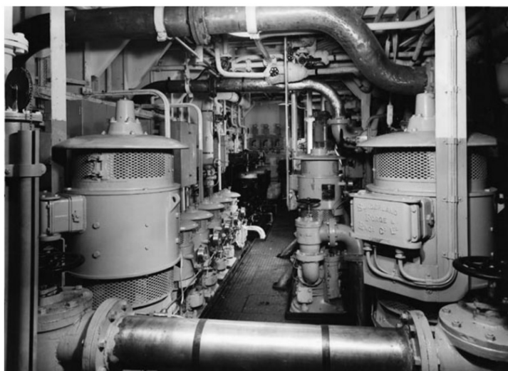
Looking aft along starboard side of engineroom, showing pumps and oil purifying equipment. Photos from the collection of the late Alec Osborne. Copyright © Reardon Smith Ships.
