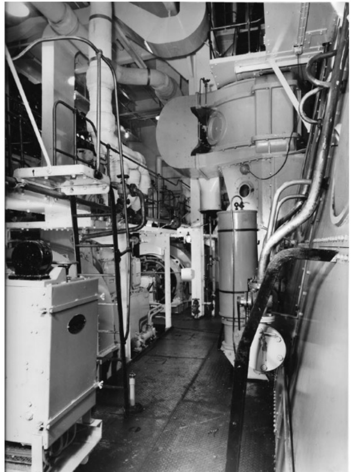
Looking aft along back of main engine. Generator gauge board in foreground.
